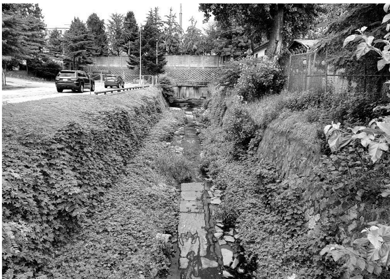
Figure 24. Water flows into Yongsan Garrison from a tunnel hidden behind metal bars and vinyl curtains. 20180706
