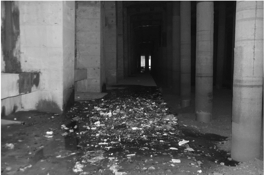
Figure 10. A pile of garbage lies beneath a grate. Daylight coming in from the river entrance is visible in the distance. 20190203
