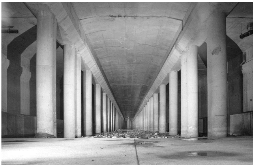
Figure 41. This stretch of tunnel under Cheongpa-ro could be renovated easily into a public park. 20130530
