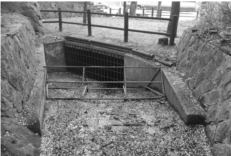
Figure 28. Up on the slope of Namsan a few meters uphill of Sowol-gil, a storm drain entrance sealed by metal bars is found. 20190421
